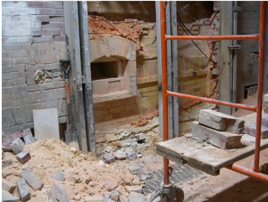
Cleaning Refractory Brick Renovation Areas where Debris of Varying Size is Generated
