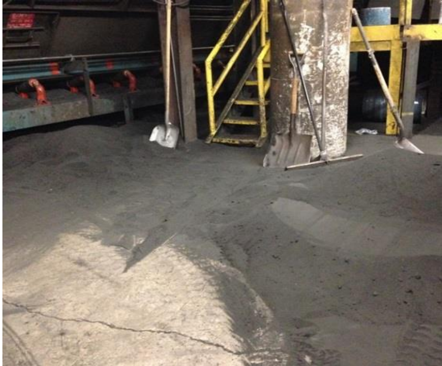
Cleaning Large Accumulations of Sand In and Around Sand Handling Systems
