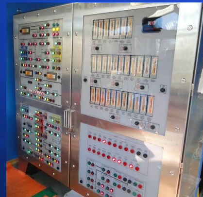
BOP Control Panel
