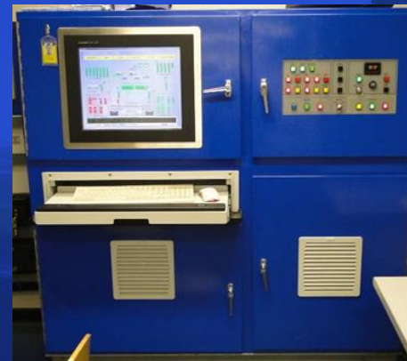
Central Control Console
