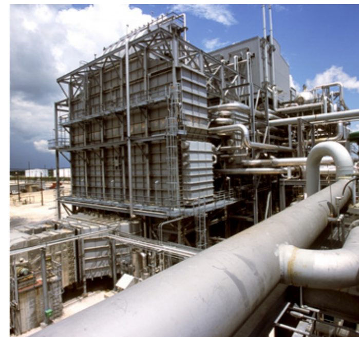
Air Products' Port Arthur Texas Hydrogen Plant. Image courtesy of Air Products and Chemicals, Inc.
